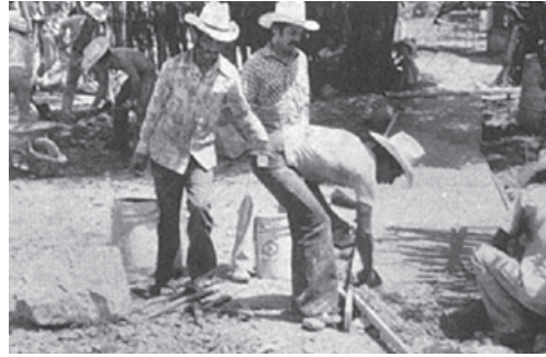
In the village of Ajoya, Mexico, over 60 families participated in building a cement walkway from the rehabilitation center to the main street.
